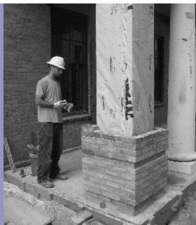
Mason provides brickwork to the new Seelos Welcome Center as the project nears completion in mid-summer! See details in future issues!
